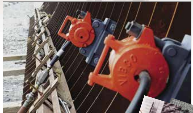
The SVRL Units shown here are being used to consolidate a concrete retaining wall. The Lug Bracket also shown, makes it an ideal solution for portability.
