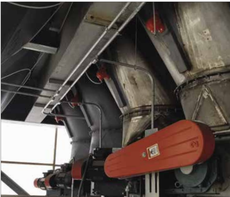
Above: The patented SVR design (page 30-31) shown in the dust collectors of this power plant, have a dB reading of 95-110. They are also available in a silent version which brings the dB down to 80-85.
